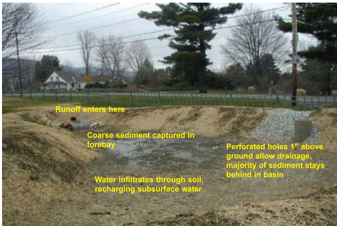
Construction of a retention basin, which is being converted into a wetland garden. It captures sediment and other pollutants.
